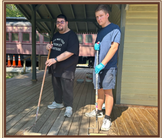
Michael Beck (left) and William Sigler (right) apply water seal to the museum deck
